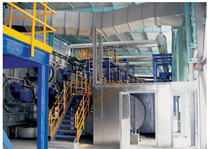
Fig. 5: Stainless steel strip floatation cooling plant with “hot cooling zone” behind the furnace
